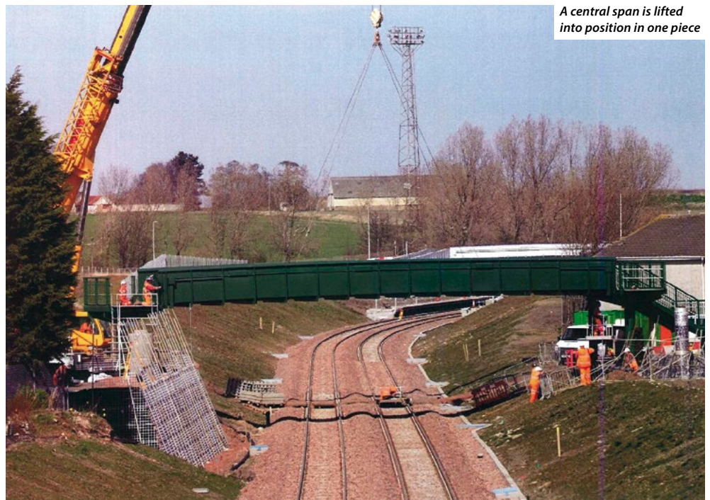
Speed of construction meant steel was the ideal material for the project's bridges
