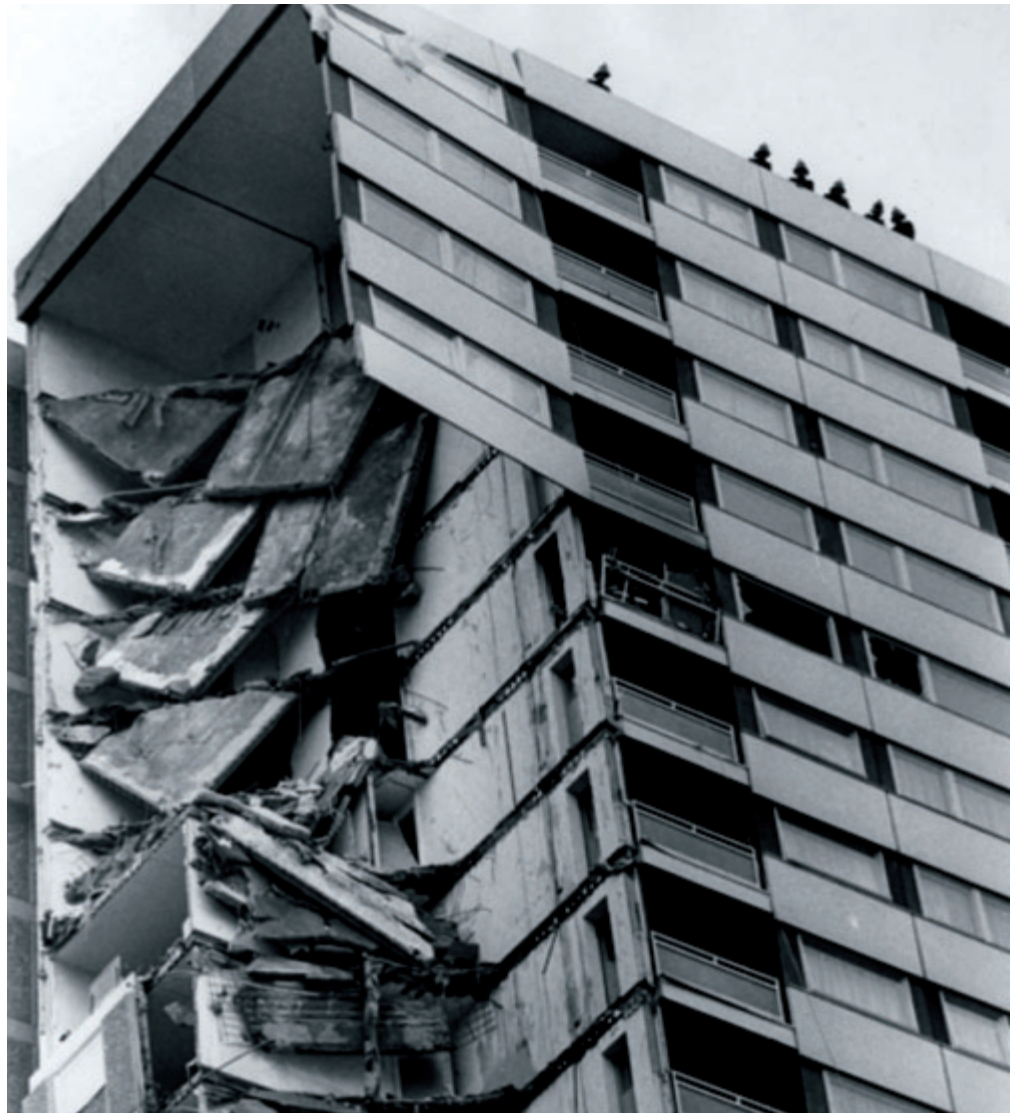
Figure 1.1 Ronan Point 1968 - Partial collapse of a concrete structure due to a gas explosion
