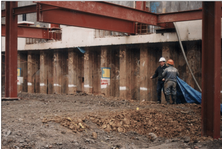
Figure 2.3 Permanent steel sheet pile wall and concrete pile cap supporting the building superstructure
