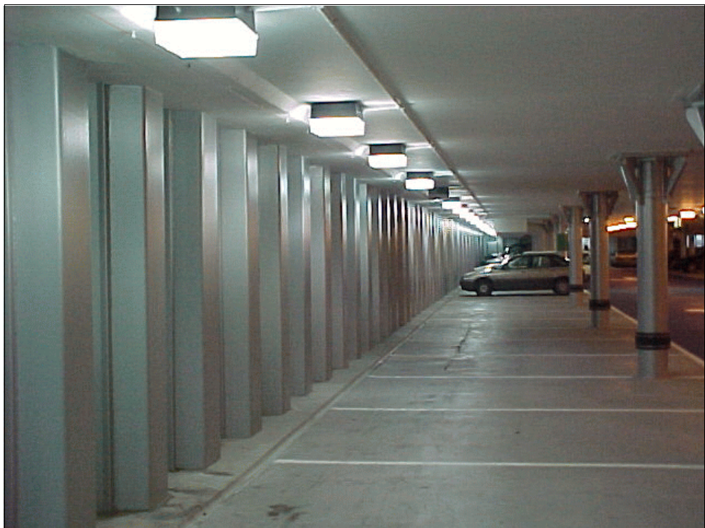
Figure 2.1 Bristol Millennium car park showing the aesthetic appearance of the sheet pile walls (see also front cover)
