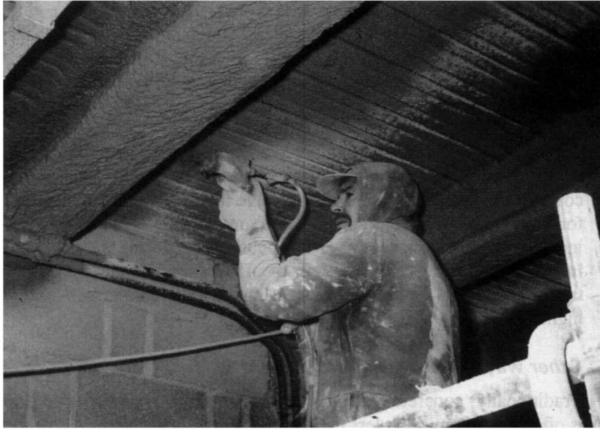
Figure 7.9 Sprayed fire protection
