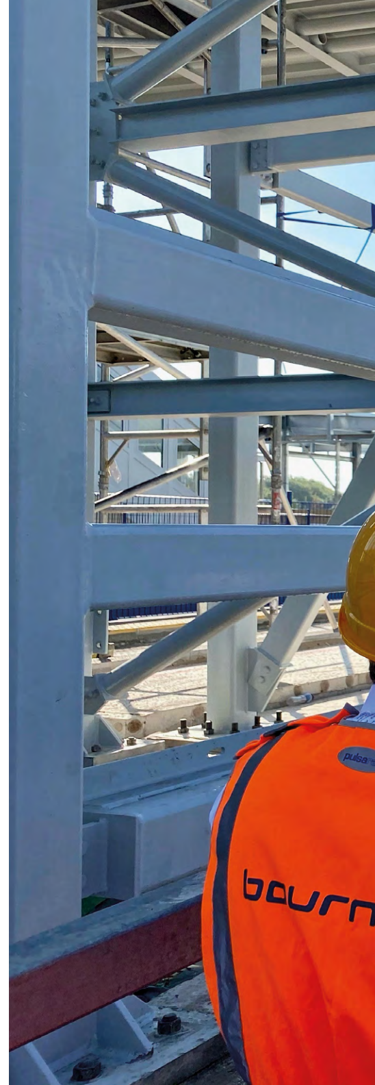
Construction work has been undertaken around a 'live' railway environment, as the station is on the busy Reading to Basingstoke line.
