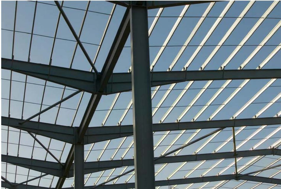
Figure 3.18 Valley beam details for “hit” and “miss” frame (Photo courtesy Kingspan Metl-con Ltd)
