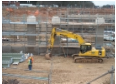
Safe site conditions
