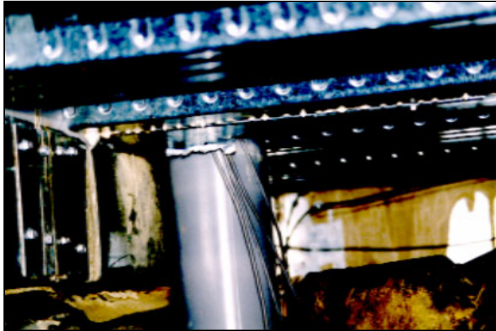
Figure 4.8 Service pipe penetrations through the steel decking, - view from void below the decking
