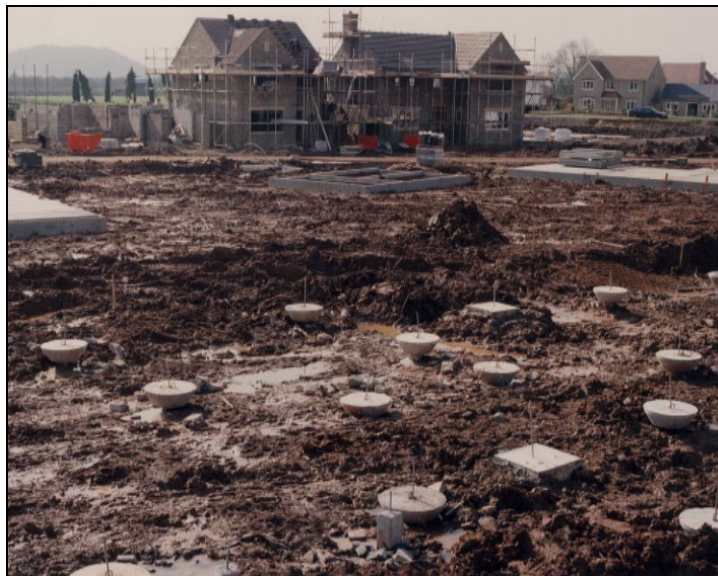
Figure 3.12 Precast concrete mini-piles on 'brownfield' site after cropping and capping (Courtesy of Bullivant Ltd)
