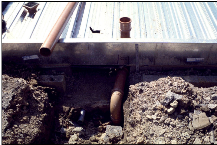
Figure 4.9 External service pipe penetrations through decking
