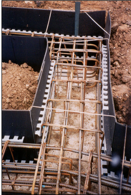
Figure 3.14 Plastic sheet formwork, reinforcement and cover strips for in situ ground beam over two piles
