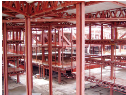
Steel structure of the main entrance hall in front of the cubes
