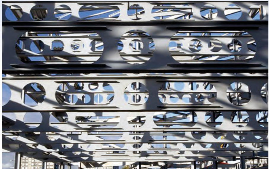
Figure 2.6 Long-span cellular beams with offsite fire protection provide for freedom in servicing
