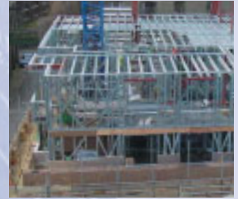
8-storey light steel Metframe construction. This minimises the load on the underlying Brunel railway tunnel, Rotherhithe.
