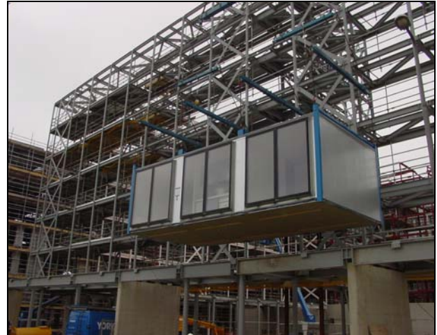
Figure 21 Installation of modules behind external steel framework at MoHo, Manchester Courtesy, Yorkon and Joule Consulting Engineers
