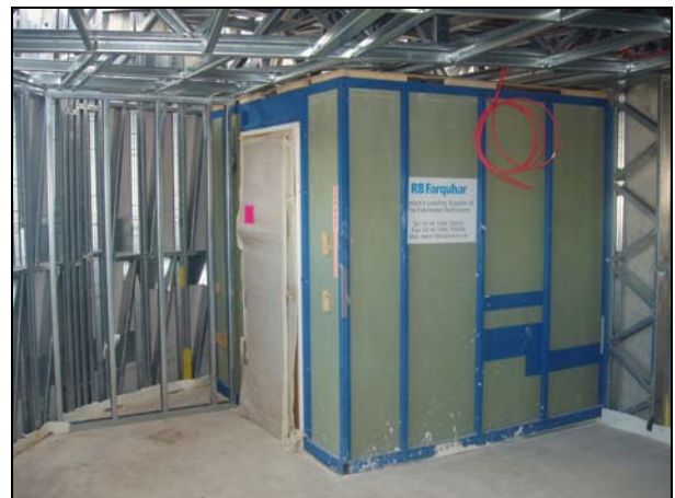
Figure 29 Toilet 'pod' used with light steel framing Courtesy, Metek UK and RB Farquhar
