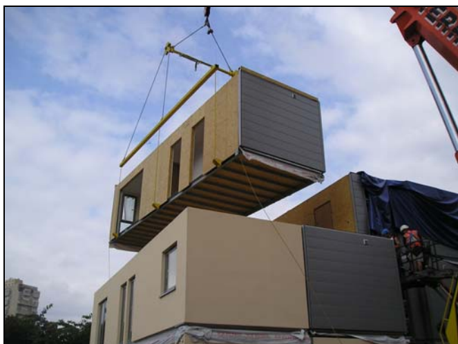
Figure 5 Partially open-ended module used in Barling Court (see opposite). Courtesy, PCKO Architects
