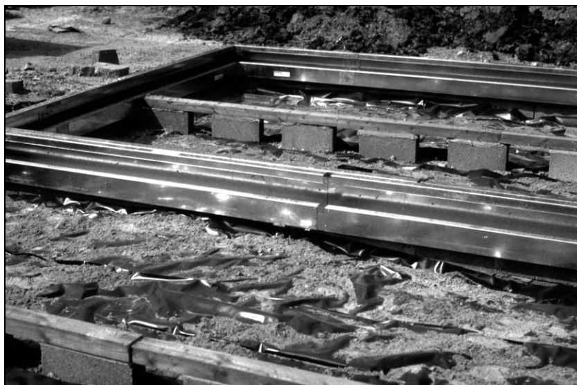
Figure 3.8 Over-site membrane applied beneath the suspended composite ground floor slab (during construction)
