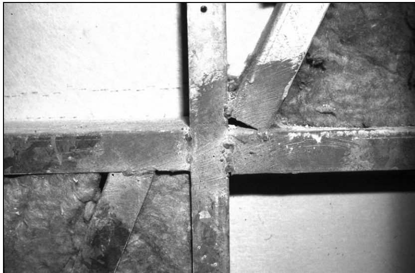
Figure 3.3 Wall panel removed, showing no trace of corrosion on the members after 14 years (the connections are coated in zinc-rich paint)
