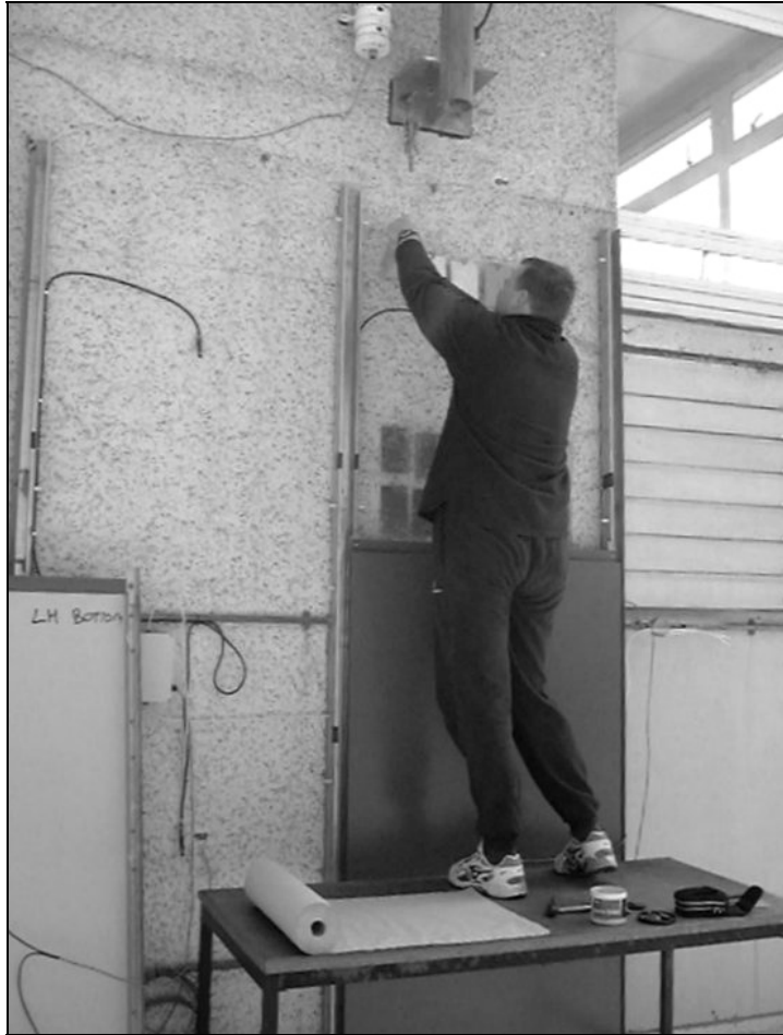
Figure 3.12 Galvanized steel coupons installed behind the steel cassette over-cladding panels in Edinburgh
