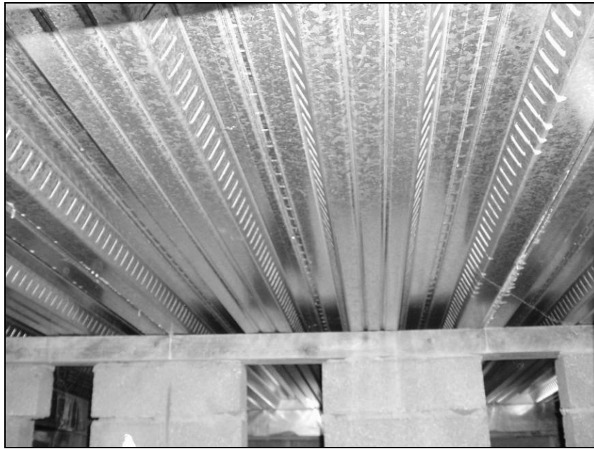
Figure 3.7 Galvanized steel decking forming the underside of the suspended composite ground floor slab after 124 months
