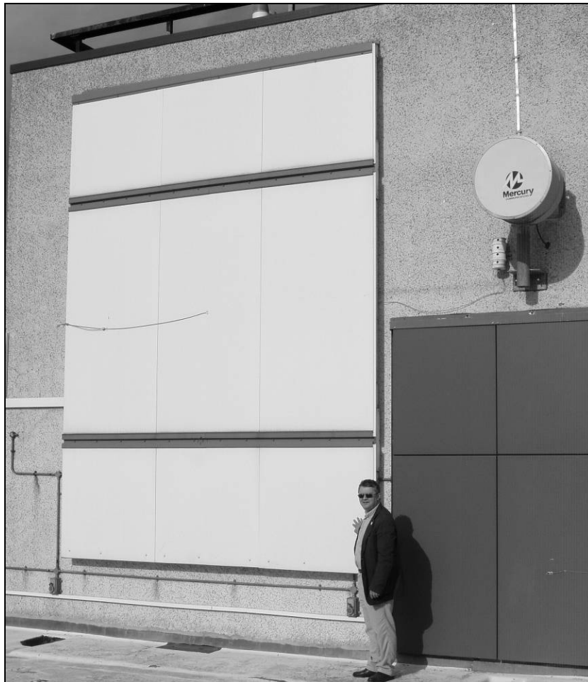
Figure 3.9 Over-cladding panels monitored on the 8 th floor of a building at Edinburgh University
