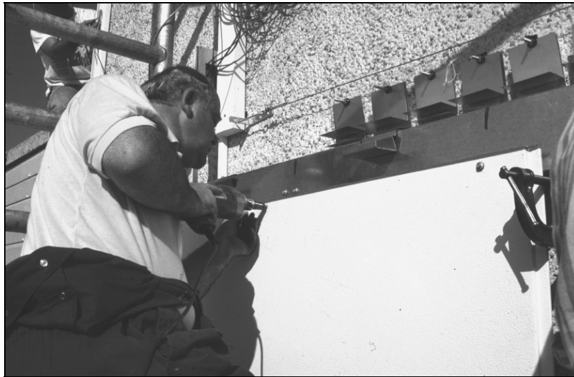
Figure 3.10 Galvanized L-shaped steel coupons installed behind the composite over-cladding panels in Edinburgh
