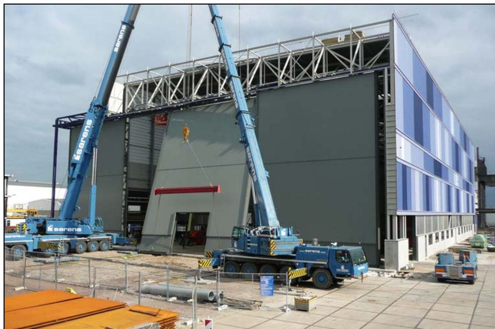
Figure 2.6 View of doors being lifted into place in Hollandia's building in Krimpen aan den IJssel
