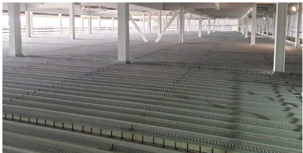
Figure 1.1 A typical example of composite floor construction, showing decking placed on a steel frame
