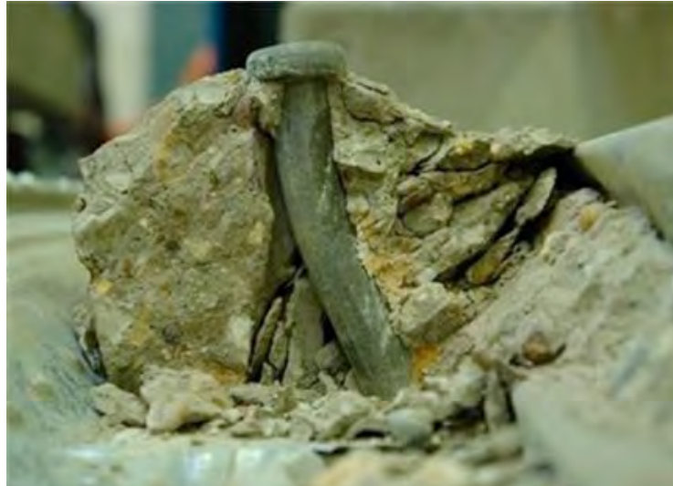
Figure 5.5 Local failure of the concrete surrounding a shear stud in trapezoidal decking
