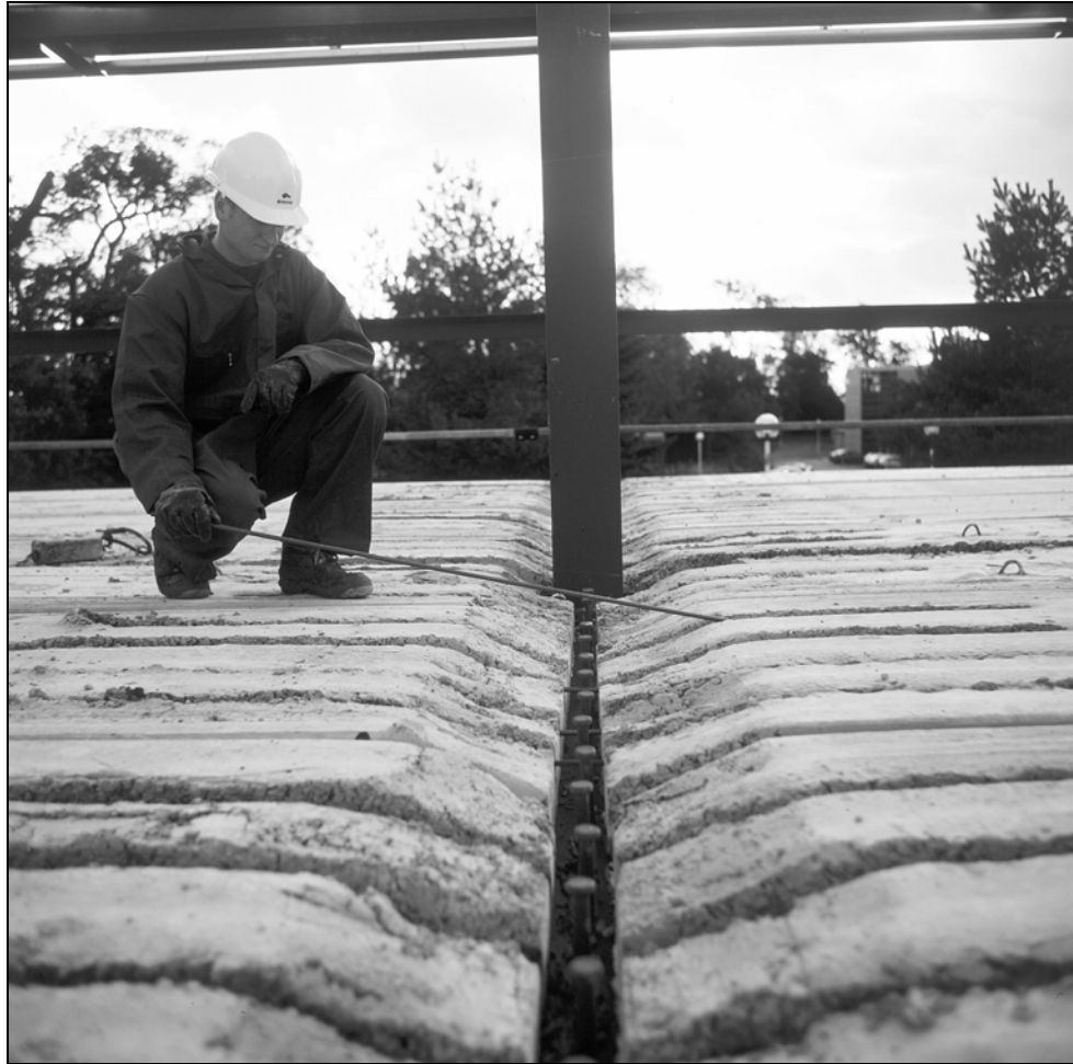
Figure 2.2 A typical example of composite floor construction with precast concrete hollow core units, showing transverse reinforcement bars being placed within the open cores
