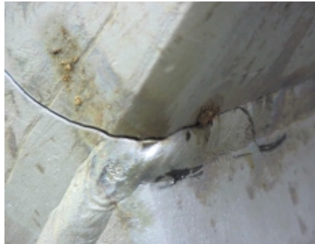
Figure C.5 Crack initiating from weld
