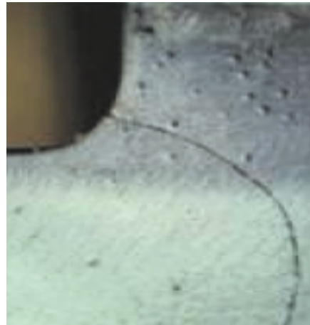
Figure C.4 Crack initiating from gas-cut corner
