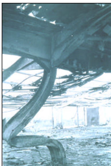
Figure 5.4 Collapse of internal column
