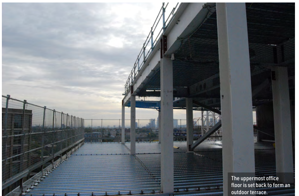
A podium column is omitted to create the main entrance and so a raking steel member, positioned above, transfers loads back into the main frame and the core.
