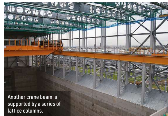
A large truss supports one of the bunker's crane beams and also spans over two hoppers.
