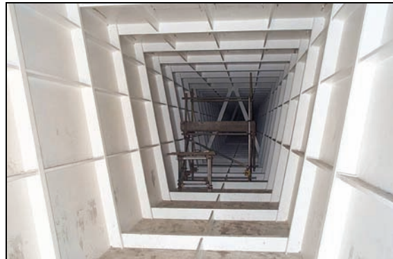
Figure 1 Internal view of a steel box girder showing use of longitudinal stiffeners
