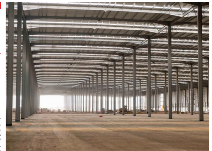
No internal cross bracing was allowed in order to maximise space inside the new M&S warehouse.
