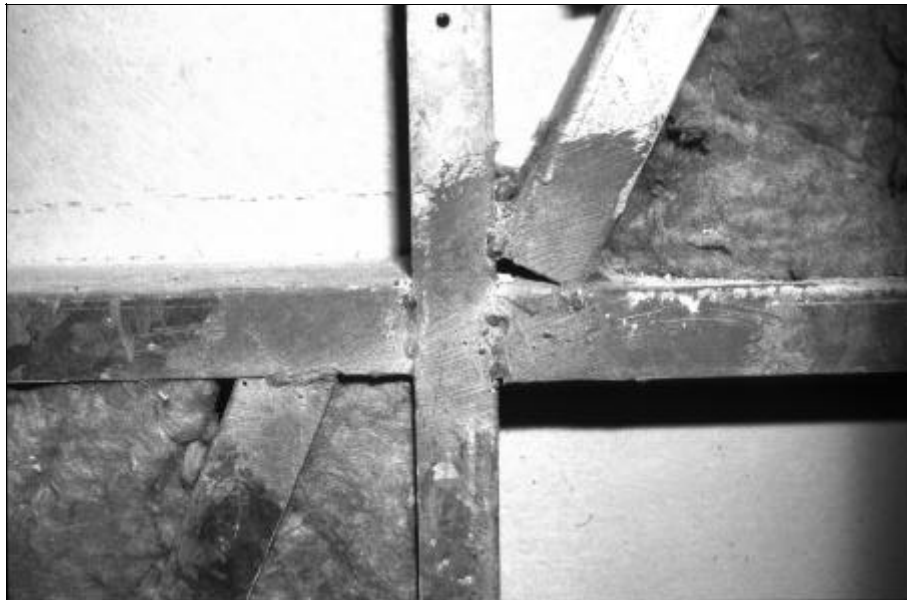
Figure 3.3 Wall panel removed, showing no trace of corrosion on the members after 15 years (the connections are coated in zinc-rich paint)
