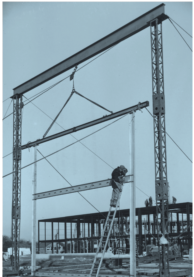
Right Slim beams and girders go up during the construction of Hunstanton School.
