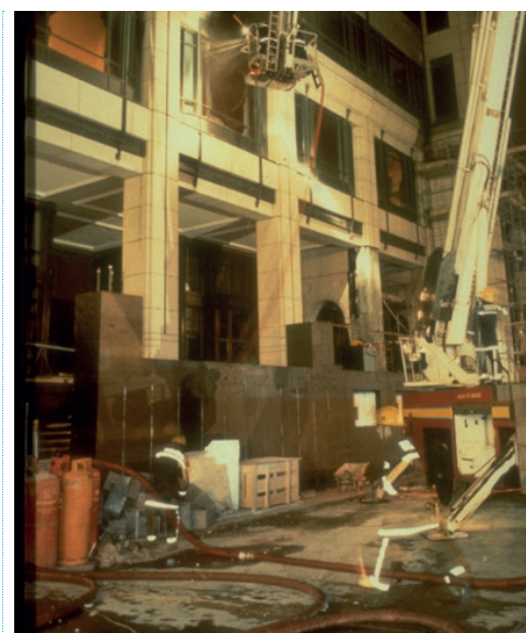
Broadgate phase 8, where a real fire in June 1990 on a partly completed structure provided useful data on the fire resistance of steel framed buildings
